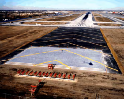
FIGURE 6: A stopway/blastpad with EMAS installed. The EMAS section is grey and slightly raised above the rest of the stopway. This example is installed on Runway 12R at Minneapolis/St. Paul International Airport, due to a deep and abrupt terrain dropoff into a river gorge just beyond the EMAS area.
