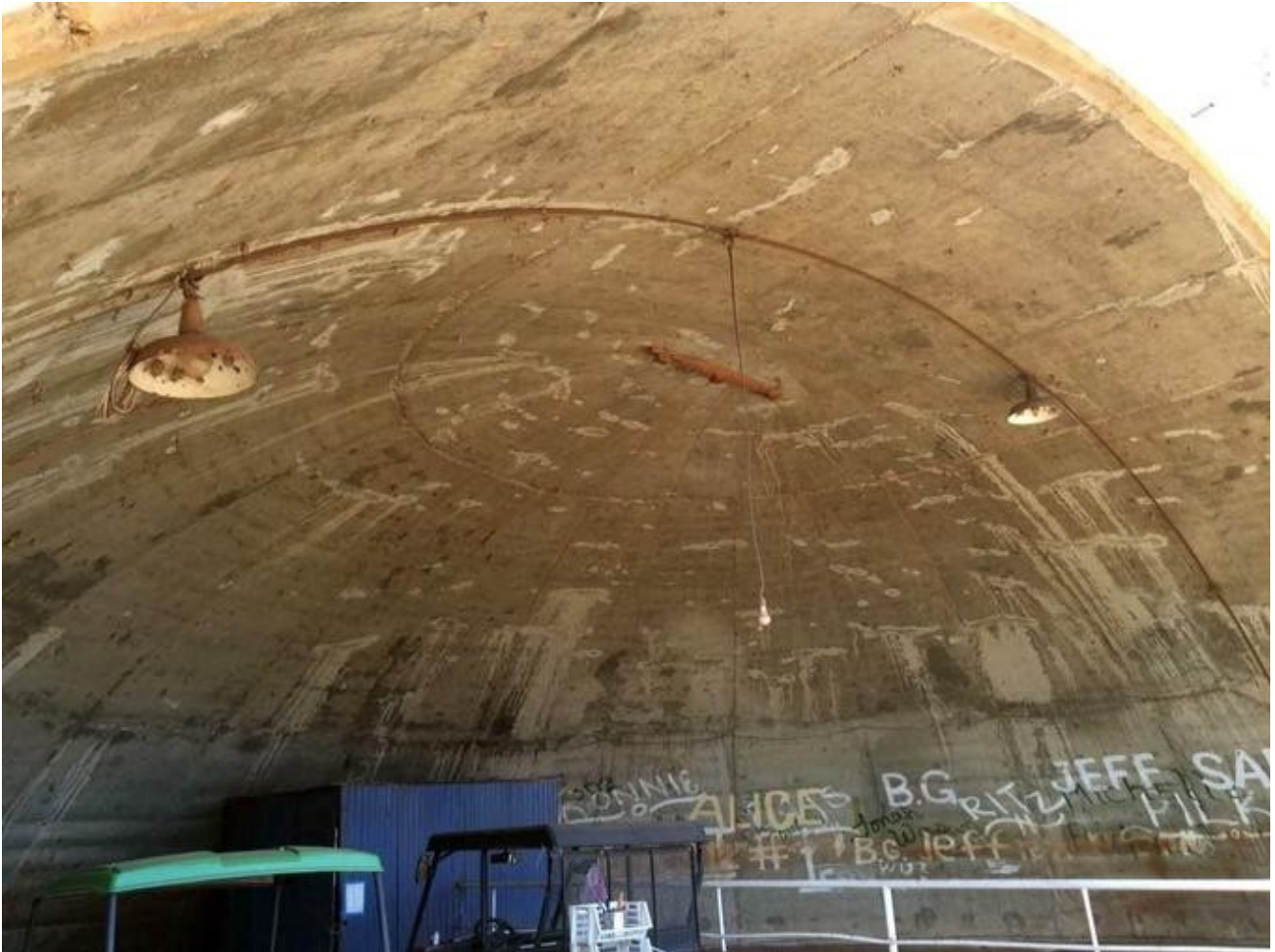
Hastily constructed revetments that protected aircraft bound for the Battle of Midway still exist today within the ruins of MCAS Ewa, O'ahu, Hawaii. [Photo Credit: via Abandoned & Little Known Airfields]
