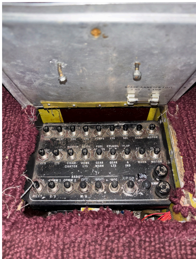
Circuit breakers recessed into the floor
